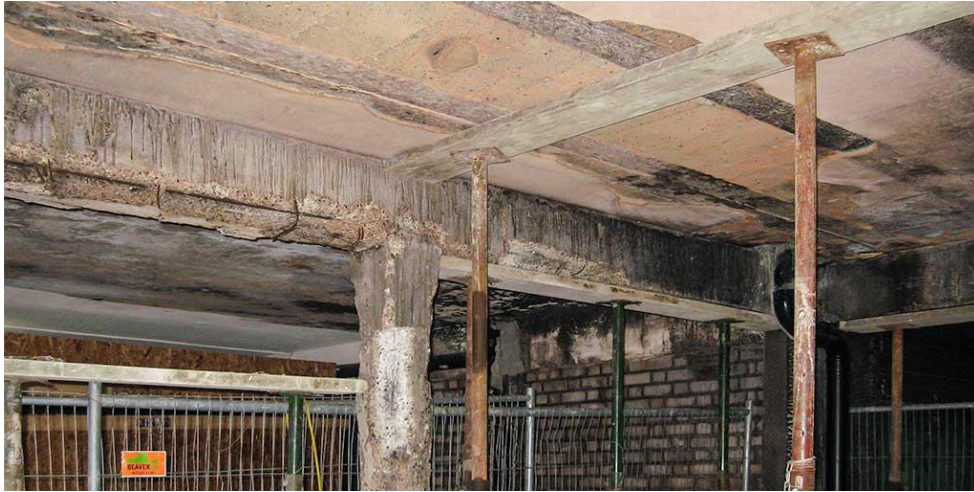
Figure 1: Damage due to Fire
